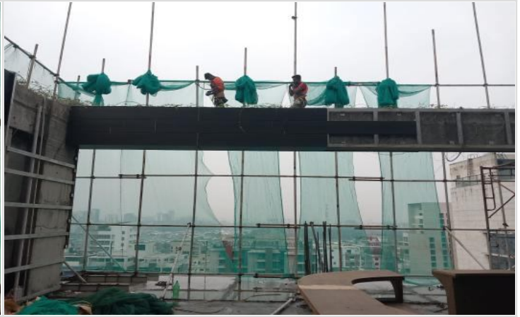
L-16-West side safety net hanging on 15-03-23
