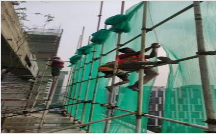
L-16-West side safety net hanging on 15-03-23
